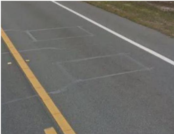
Traffic Monitoring System
